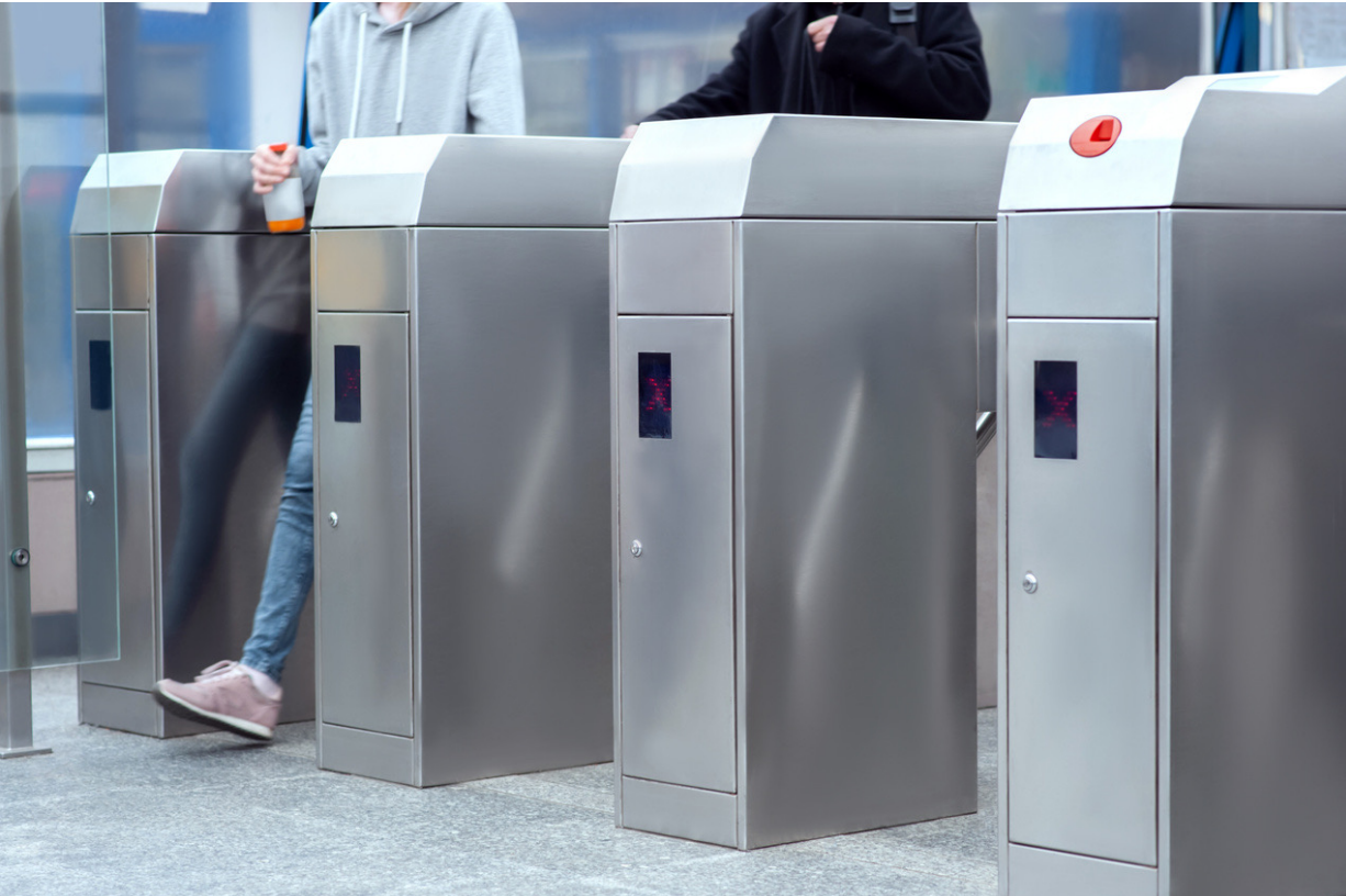
AFC (Automatic Fare Collection) System
